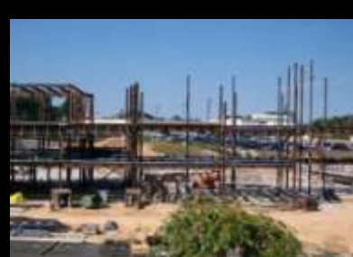
This is the view from Carver's roof of the new main entrance now under construction.
